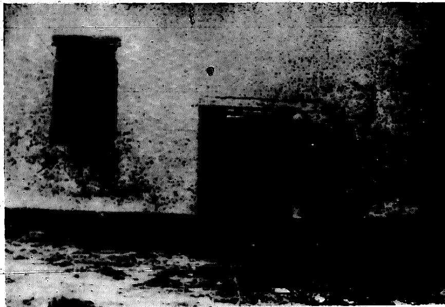
Figure 27. A soil bearing failure has caused structural cracks in the foundation footing wall and the adobe wall in this large community building.
